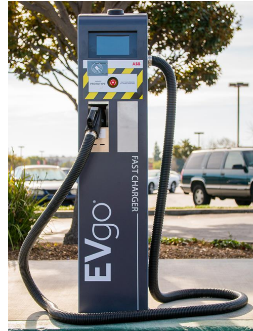
350 kW-capable DCFC deployed in Fremont, CA
