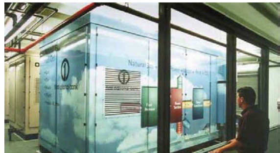
First National Bank of Omaha puts the cost of outages at its credit card processing center, seventh largest in the nation, at $100,000 per minute. Such high-stakes risks are driving the growth of distributed energy installations such as this fuel cell array at the Omaha center.
